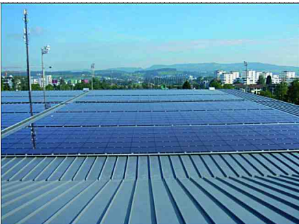
204.4 kWp Bossard Arena Zug
