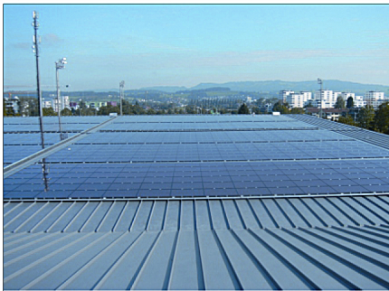
204.4 kWp Bossard Arena Zug
