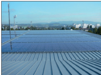
204.4 kWp Bossard Arena Zug
