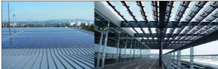
204.4 kWp Bossard Arena Zug
